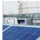
ITALY Cooling loop flow & temperature control
