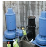
IRELAND Maintaining pressure at pumping stations
